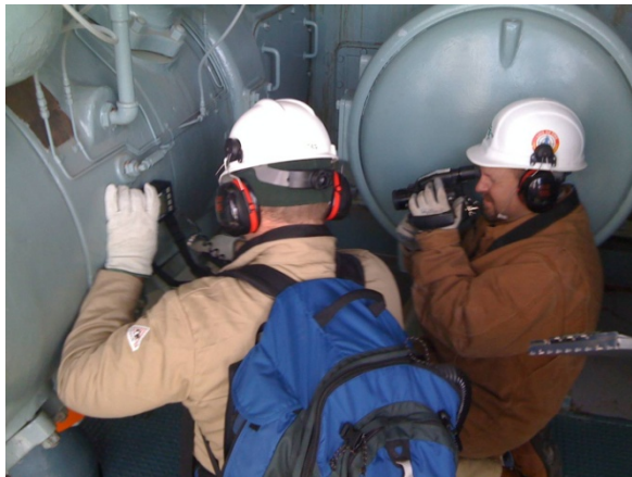
Figure 2-3. FLIR Camera (right) and Hi-Flow Sampler (left)
