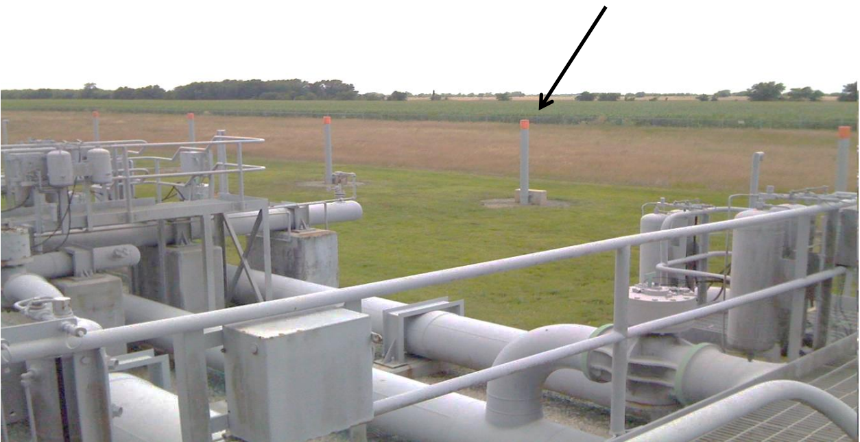
Figure 1-2. Compressor Blowdown Vents
