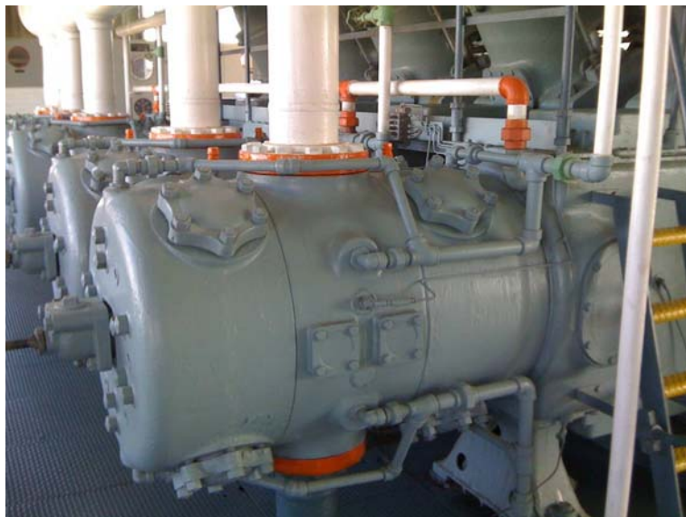
Figure 1-6. Reciprocating Compressors (note the 2” rod packing line with orange elbows)
