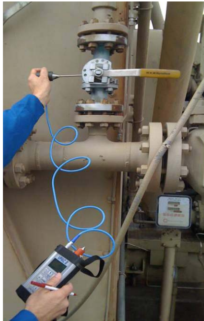
Figure 2-6. Through-Valve Acoustic Leak Detection (VPAC)
