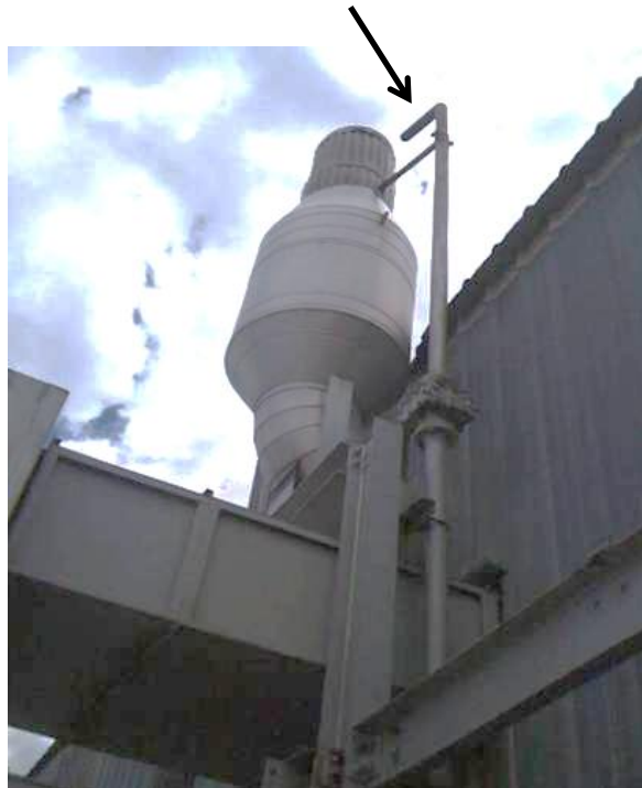
Figure 1-1. Centrifugal Compressor Wet Seal Degassing Vent
