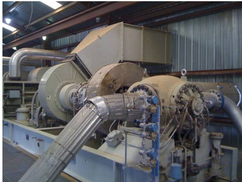
Figure 1-4. Centrifugal Compressor (foreground) with Turbine Driver (background)
