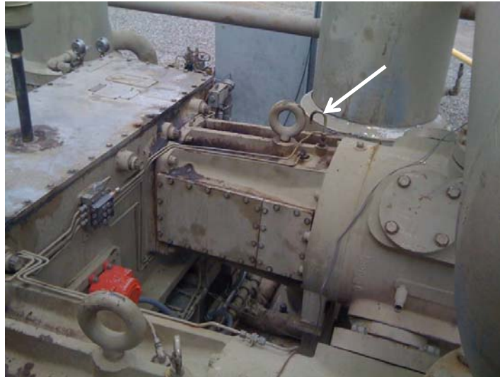
Figure 1-7. Reciprocating Compressor Rod Packing Vent (Gathering Service) (1/2" tubing)
