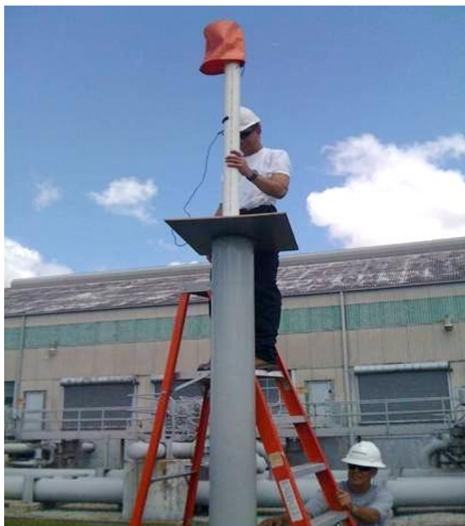
Figure 2-4. Measurement of Compressor Blowdown Vent Line Leakage with Encased Rotary Vane Anemometer
