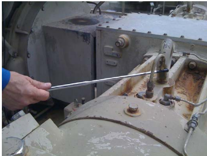
Figure 2-8. Sampling a Rod Packing Vent with Hand-held Hot Wire Anemometer
